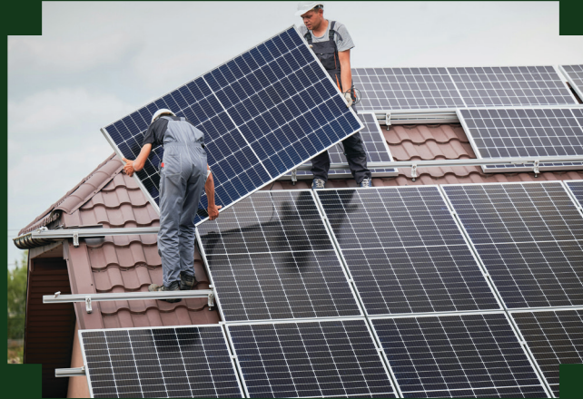
SOLAR PANELS WITH BATTERY STORAGE AND AIR SOURCE HEAT PUMP
