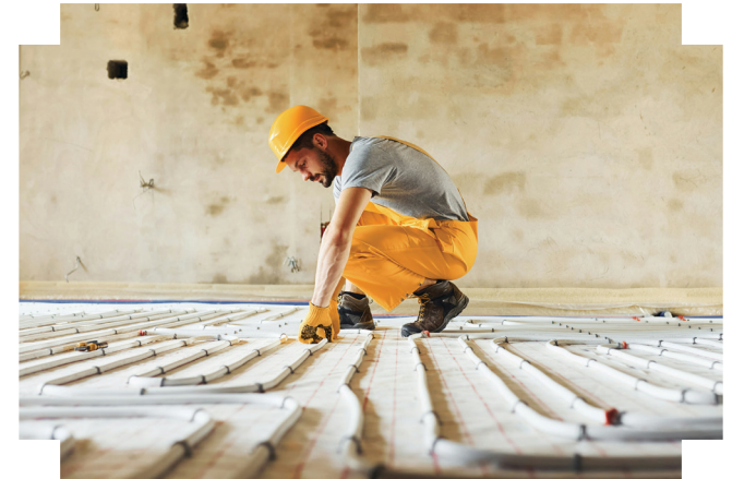
UNDERFLOOR HEATING TO THE GROUND FLOOR
